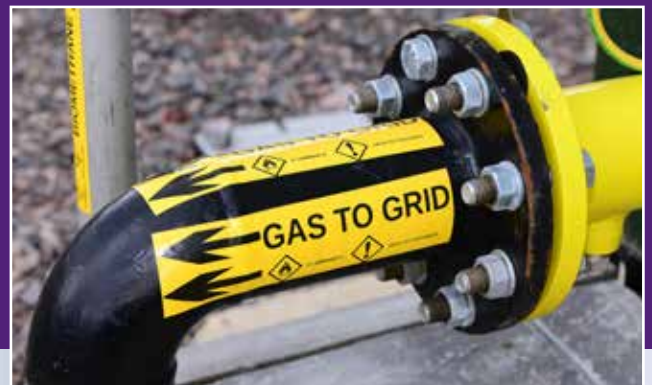
Upgraded methane is injected directly into the national gas grid
